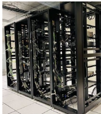
Liquid cooling rack system built from ground up with CDUs and underfloor manifolds.
